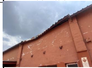
Damaged section of roofing
