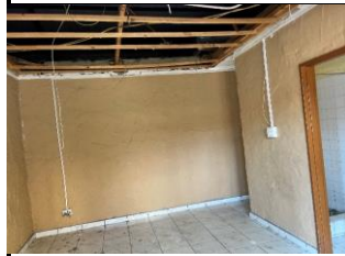
Accommodation suite with missing ceilings
