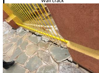
Crack at retainer wall
