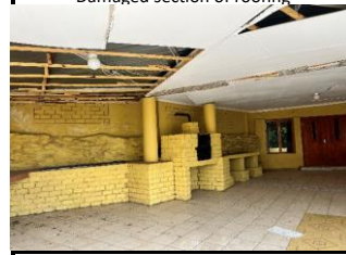
Entertainment with some missing ceilings
